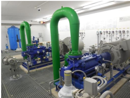
Grubbach combined pump- and hydropower station
